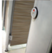
Fixings concealed from exterior view
